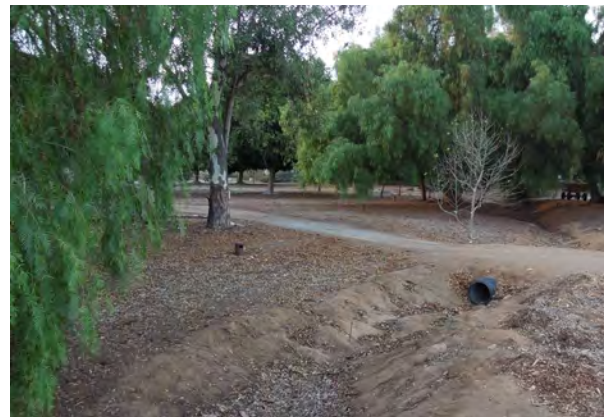
Drainage Ditch at Cuyamaca College Lacks Storm Water Treatment
